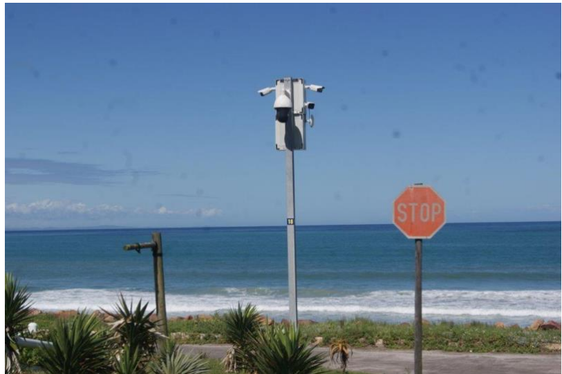
Figure 2 Typical CCTV pole
